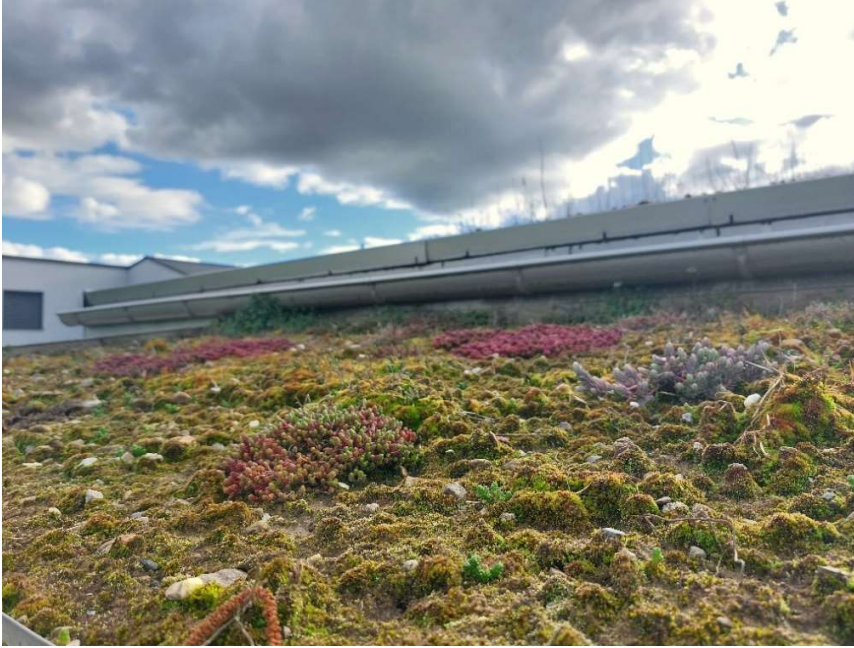
Fig. 6 Example of an ultra-extensive green roof with a 5 cm layer of topsoil substrate, colonized by mosses and some vascular plants ( Sedum ). Situation 2 years after installation.
