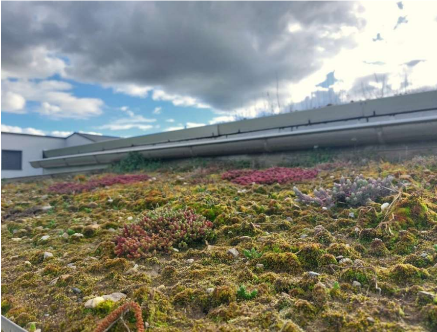
Fig. 6 Example of an ultra-extensive green roof with a 5 cm layer of topsoil substrate, colonized by mosses and some vascular plants ( Sedum ). Situation 2 years after installation.
