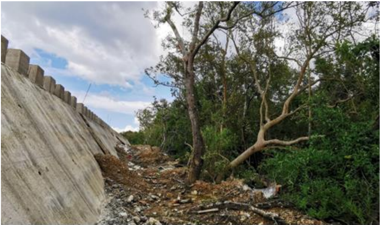
Mangrove forest destroyed during coastal road construction in Marinduque Province, Philippines (Photo credit: Dixon Gevaña).
