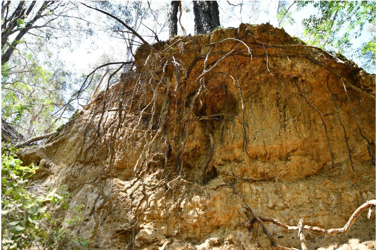
A number of sections along the northern bank of the western arm of the creek are experiencing severe erosion; here, the top of the bank is 3–4 m above the water.
