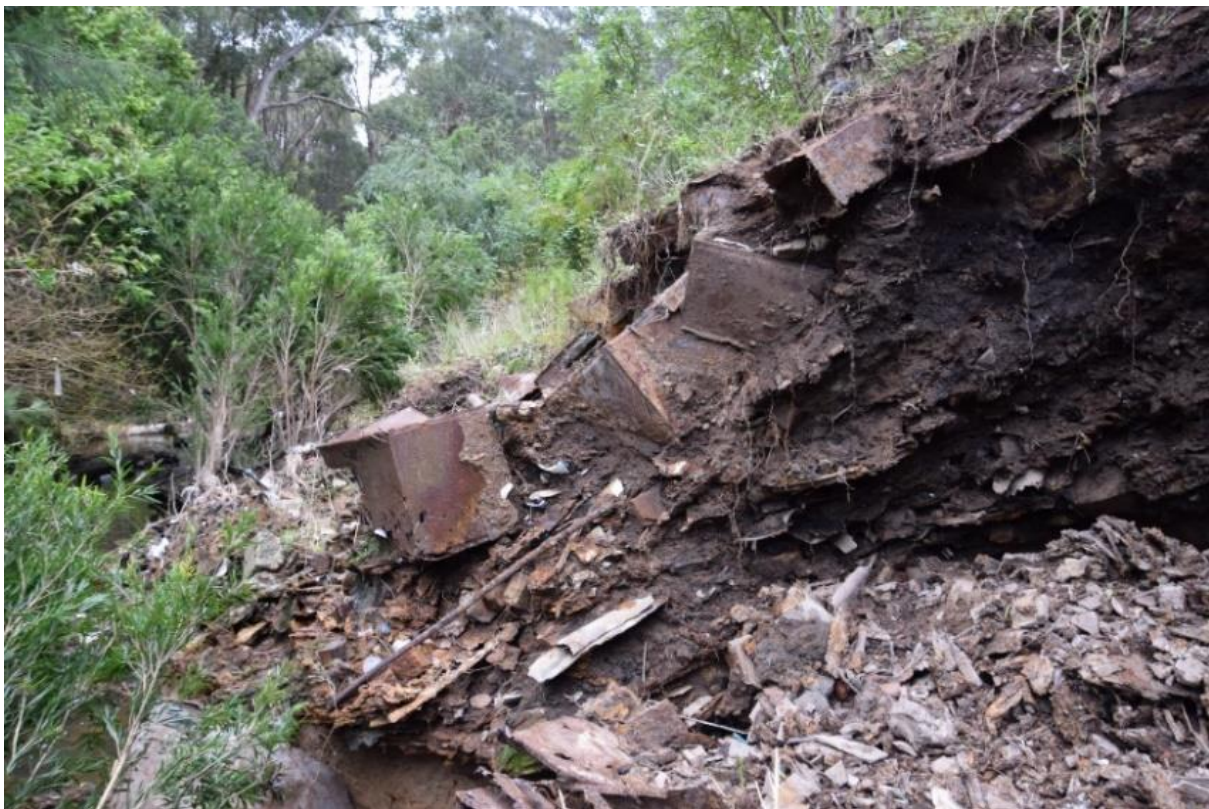
A section of the eastern bank that, having already started to strongly erode, had large sections swept away during the heavy rains and flooding in mid to late March 2021, exposing large quantities of industrial waste and debris.
