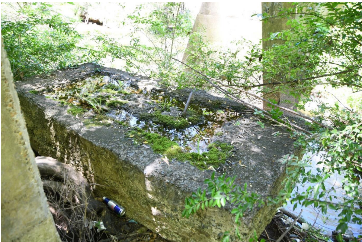
The ephemeral pool on the broken concrete pillar underneath the creek-spanning pipe, an important microhabitat for a number of aquatic invertebrates.
