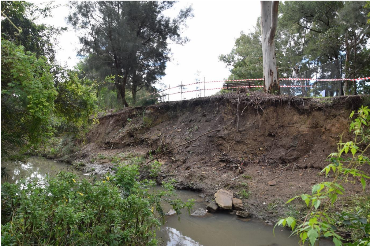
Heavy erosion on the eastern bank of Duck River, along the edge of Auburn Golf Course.
