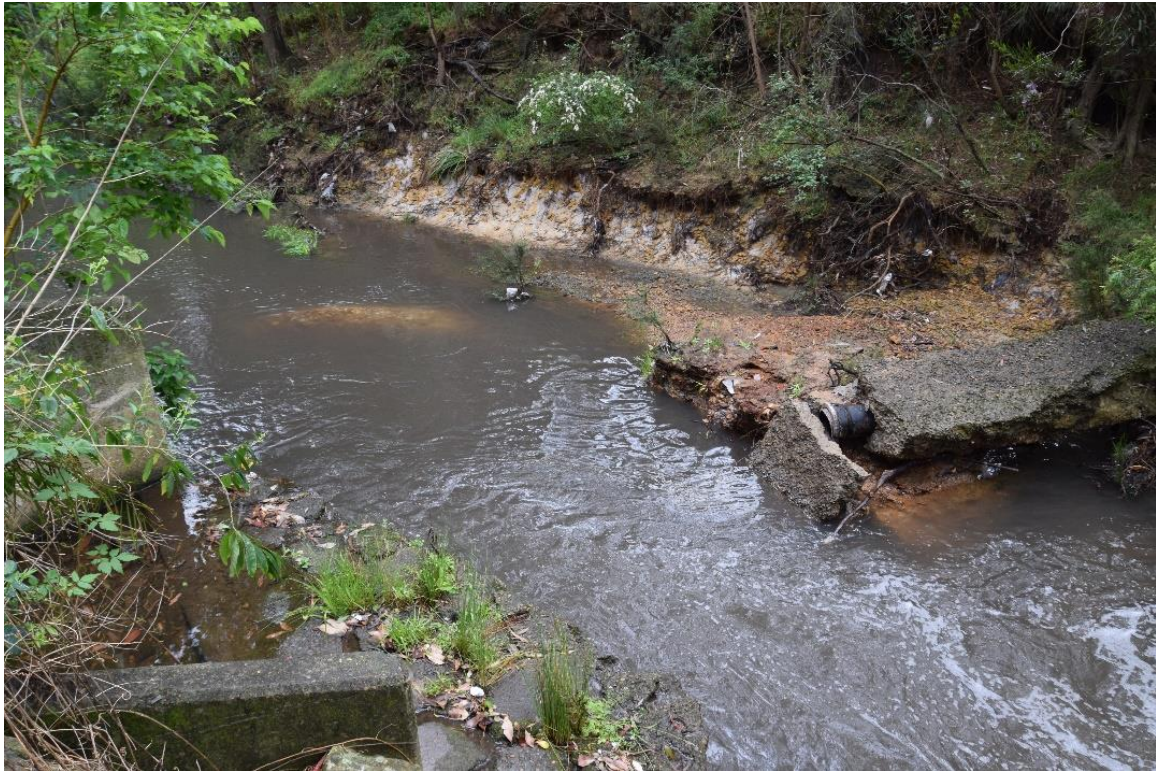
The concrete bridge just north of the creek crossing, having broken and toppled into the creek sometime in early October 2021 after heavy rain.
