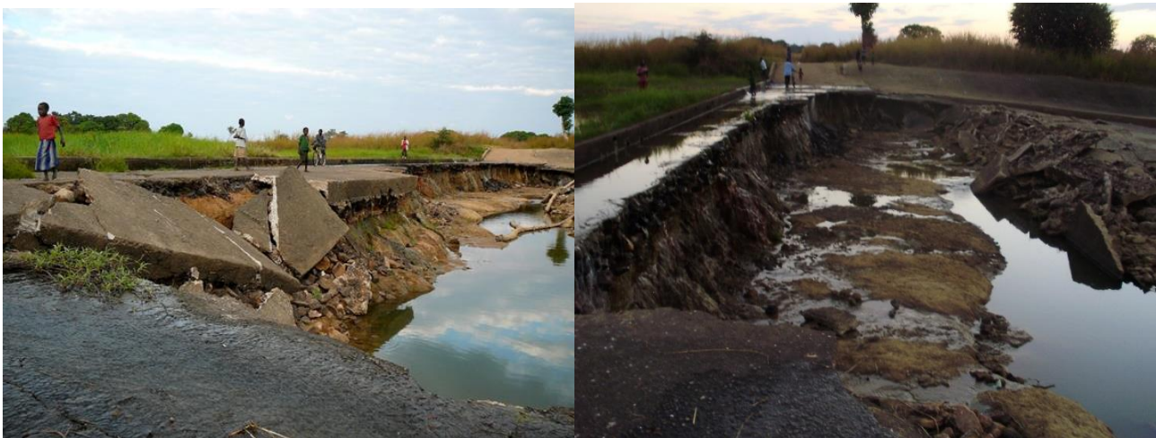
Figure 9. The crumbling dam wall of Lake Chilingali in 2009.
