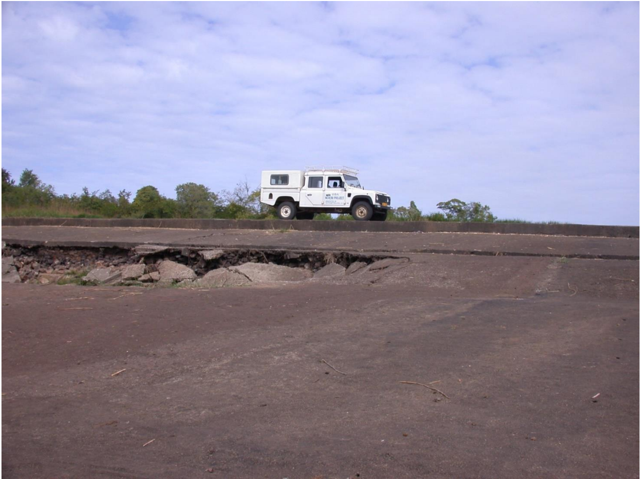
Figure 8. Lake Chilingali, the dam wall showing signs of erosion in 2004.
